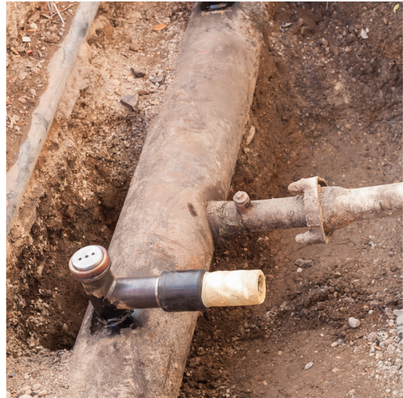
Water Main & Water Service Line
